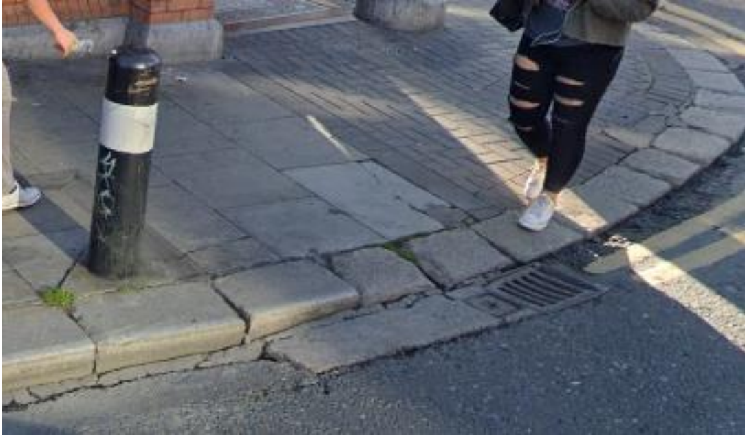
Figure 40: Drainage example of deterioration, both of the kerb and adjacent gully.
